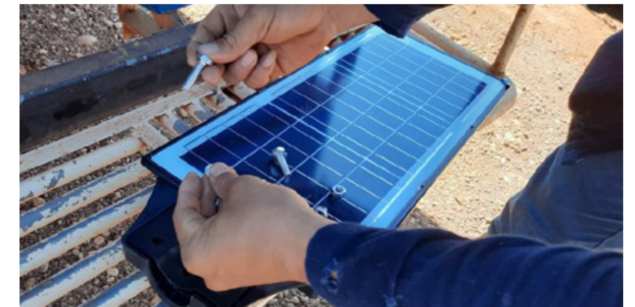
Employees preparing to install solar panel street lights on a bridge with no lighting (Savannakhet, Laos).
